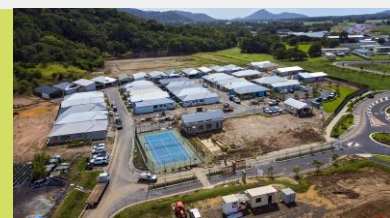
Cover: Construction progress at Botanica Lifestyle Resort by Paul Furse/ Front Row Foto
